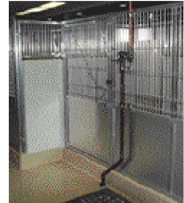
flush drains in the kennels
