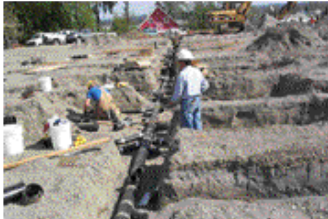
Six-inch drain pipes underneath the kennels
