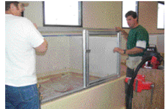
Installation of the puppy kennels. Notice the raised height of the kennels.
