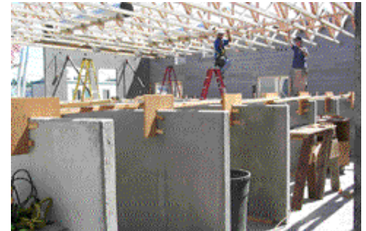
Construction of the kennels. The pre-cast panels separating each kennel can be seen in the foreground.
