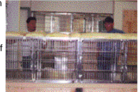
Installation of the double-sided cages in the cattery. These allow for ease of access by the staff and for maximum ventilation benefits.
